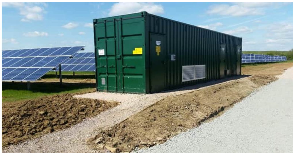
Plate 5. Typical unit housing the transformers and switchgear
