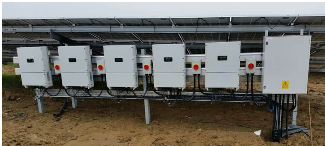
Plate 3. Typical string inverter installed next to PV modules
